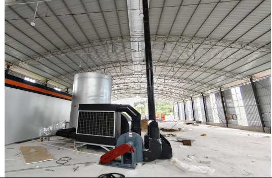
1#热风炉+1#水膜除尘器+DA001
